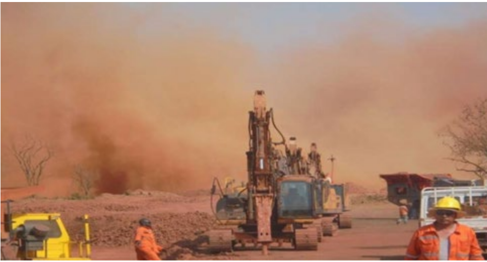
Figure 4. Air pollution related to blasting bauxite mining (Source: Author's field work, 2016)
