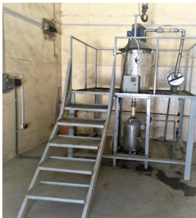
Figure 2. Steam distillation plant (Source: Authors)
